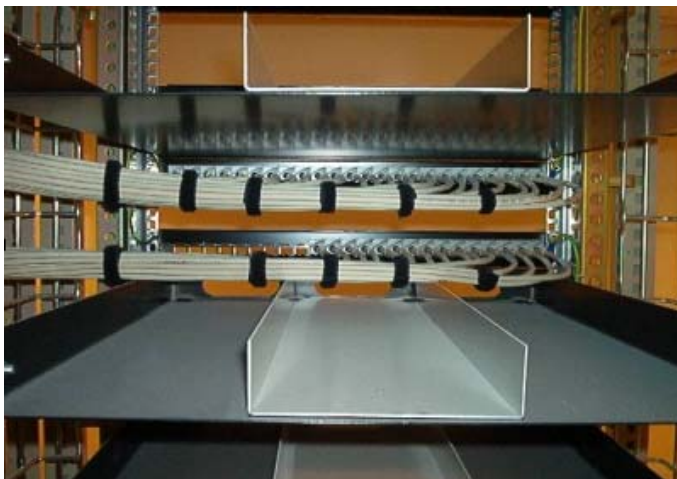
Patch panel cabling
